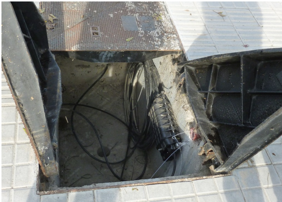
Figure 15: The cable follow the street advancing underground. One bunch of fibers turn to the left, the other bunch continues straight.
