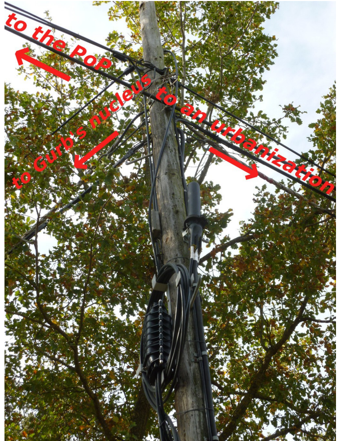
Figure 14: A bifurcation of the cable from the PoP. One goes to the urban area of Gurb, and the other to a residential area.
